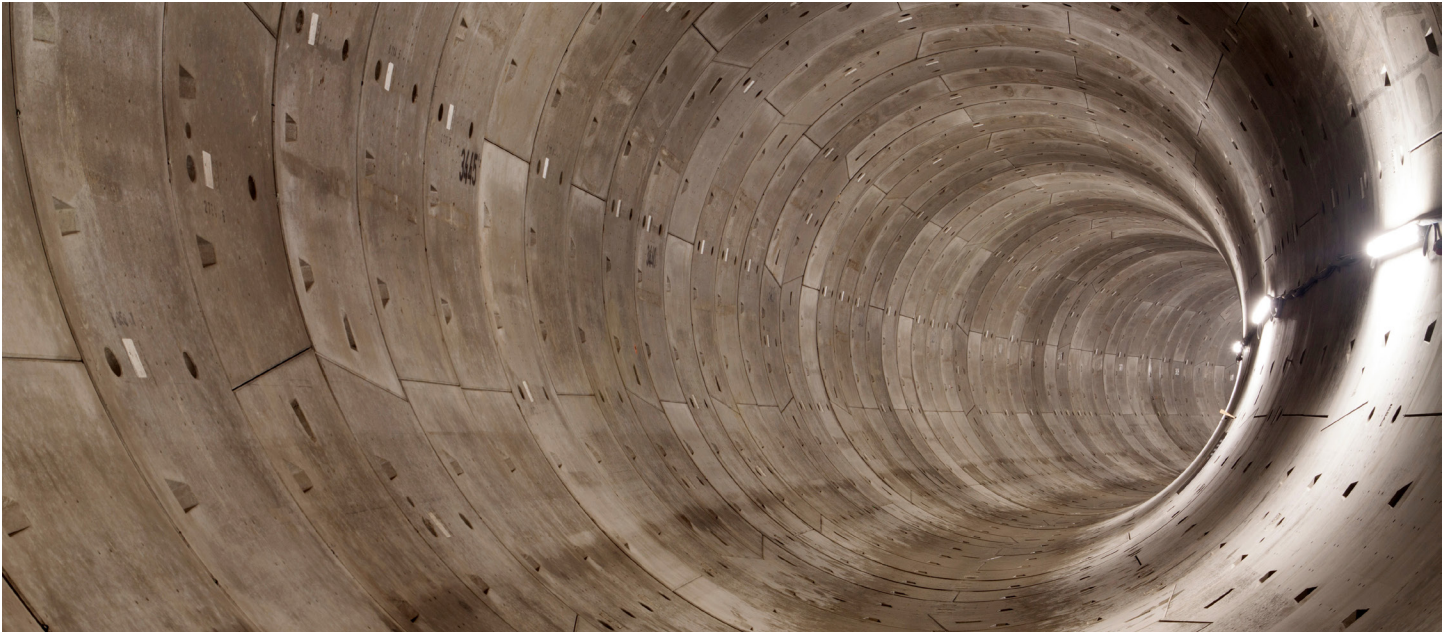
Interior view shows the cement segments that are designed to give a tunnel better seismic resilience than an above ground structure.
